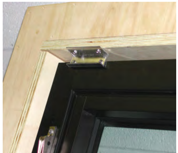
MAKE SURE WINDOW IS TIGHT TO PANNING AND INSTALL CLIPS OR TRIM
